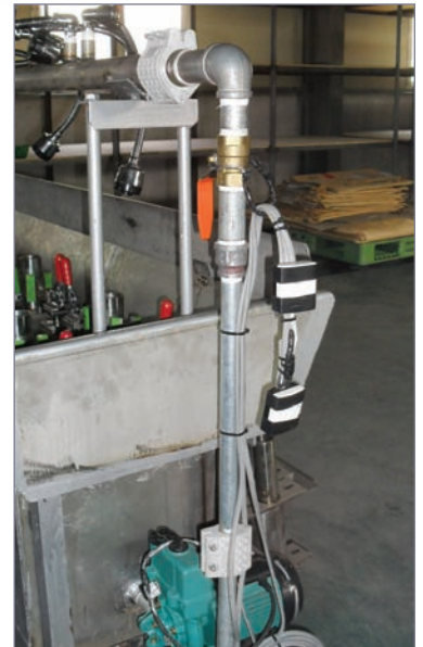
Pipe for machine with severe vibration
