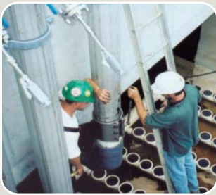
▲ Canada: water purification facility
