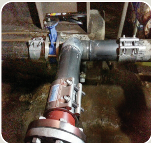
▲ Netherland desalination treatment facilities
