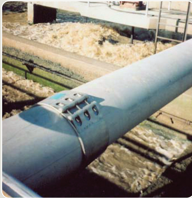
▲ Spain: water purification facilities
